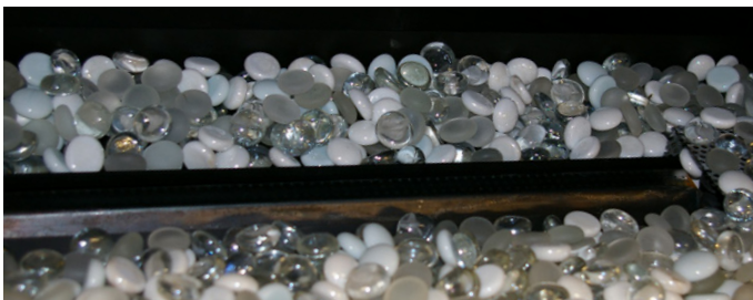
Figure 30a. Completed firestone installation. Second Gen burner shown.
