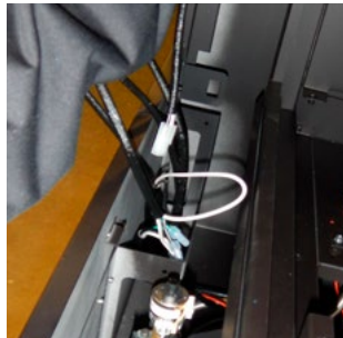
Figure 24.f Fan, LED, PPO, and pilot wires through drawer
