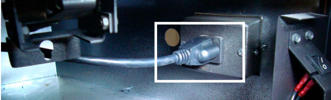
Figure 3 Powercord in PPO box
